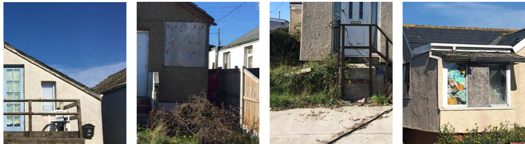
Fig. 49. Examples of occupied housing in poor condition.
