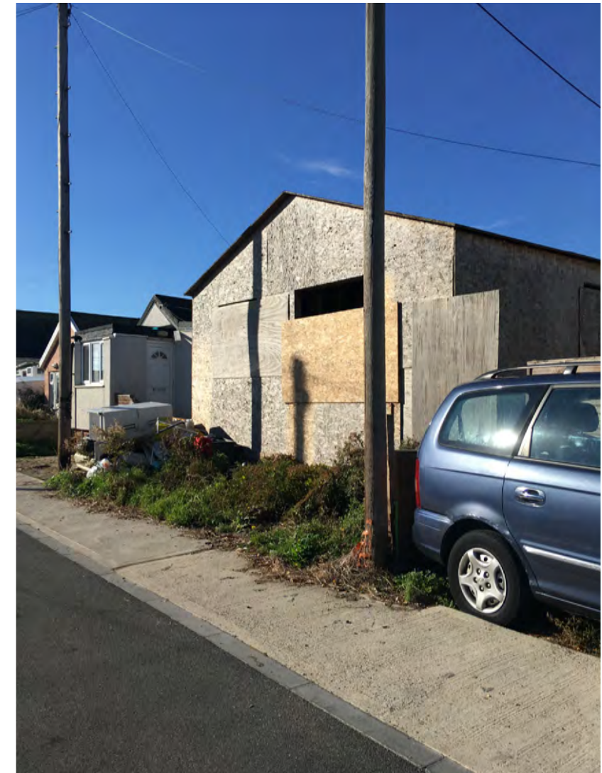
Fig. 50. An example of vacant and derelict housing in poor condition.
